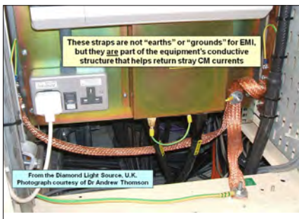
Figure 13. ... these are also not “earths” or “grounds” for SI, PI or EMI.
